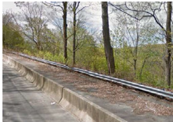
Development along Waterville Street's steep slope has led to road washouts and costly repairs. Future development on steep slopes should be subject to special development requirements © Google Maps
