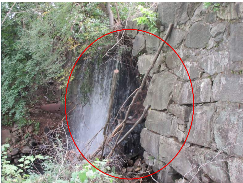
Photo 2 – Partially failed section of dam adjacent to spillway
