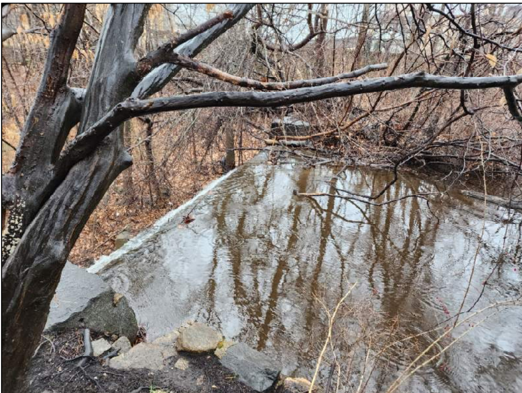
Photo 4 – Overview of spillway weir; note sediment level is just below the weir
