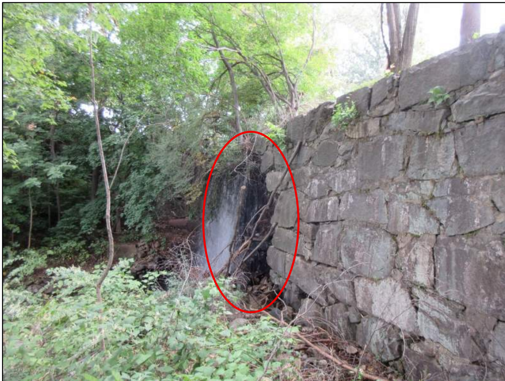
Photo 1 – Overview of downstream face of dam from south end; note partially failed section circled in red
